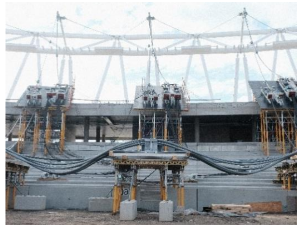
Figure 6 The cables before the strain
